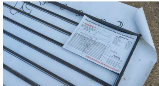
Parts laid out on the scale drawing with the measurement specifications for a panel ▶
